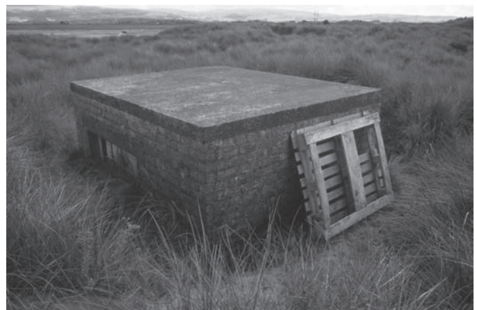
Fig. 5 Ynnyslas, Dyfed, wartime observation post for the remote filming of test firings. (© Wayne D Cocroft)
