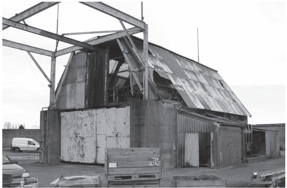
Fig. 23. Westcott, Buckinghamshire, Stand E originally built for testing Blue Steel's Stentor engines, Listed Grade II. (© Wayne D Cocroft)
