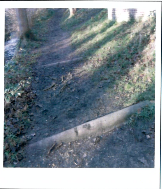
Coping of the scoop culvert walls still visible next to the tower
