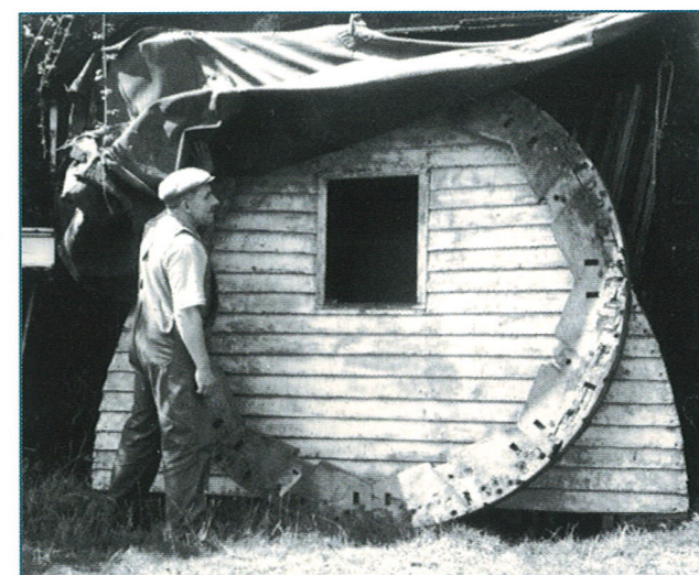
Suffolk millwright Jesse Wightman reveals components removed during the repair of Saxtead Green post mill
