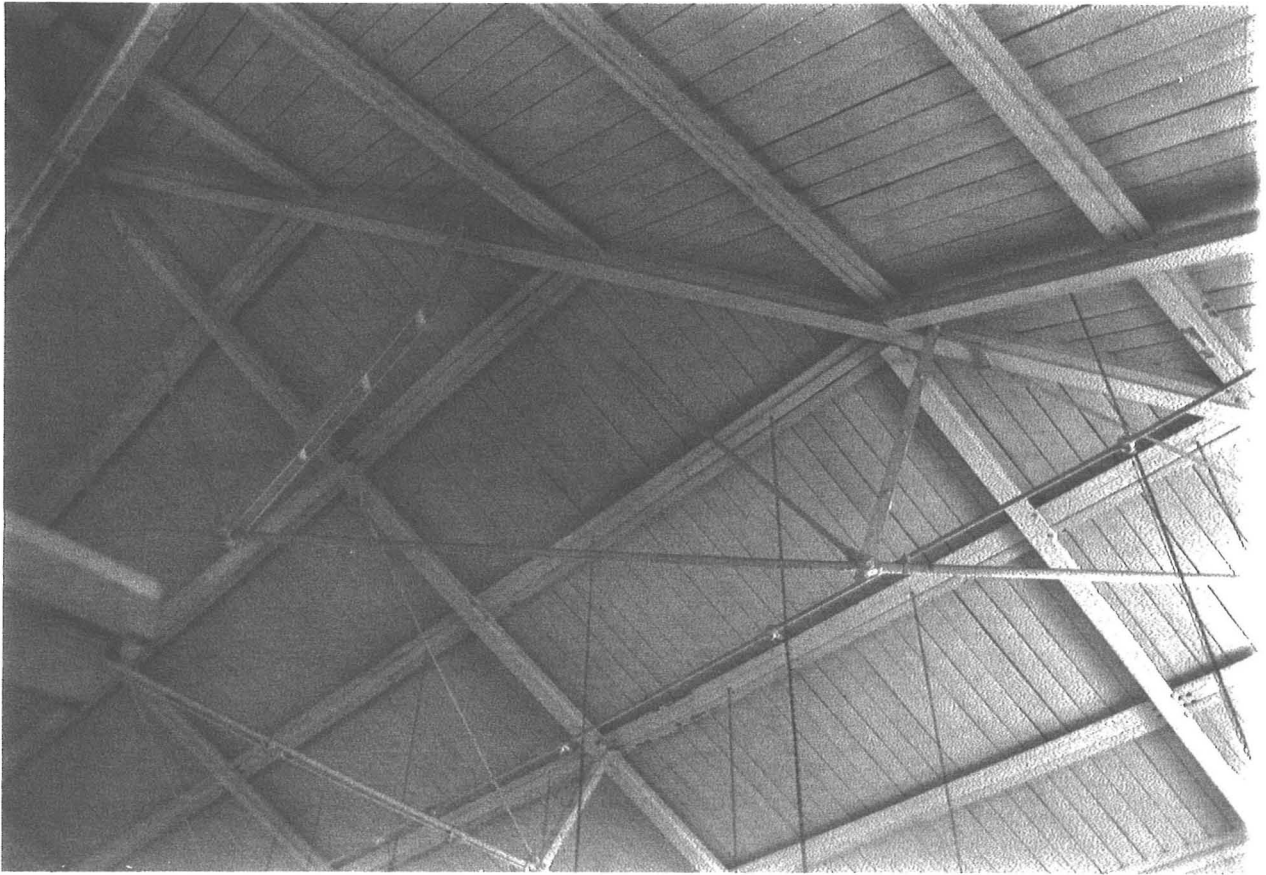
G431 PLATE 34 - ROOF TRUSS, NORTH EAST CORNER. NOTE THE BENT HANGER
