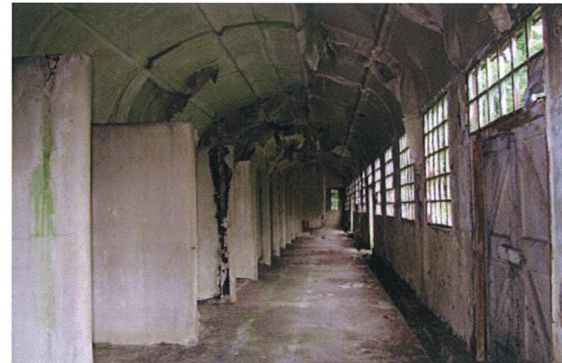
The interior of the Quinan Stove, with its series of drying bays (left), showing the now degraded condition of the interior
