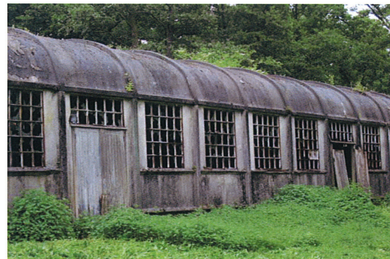
Detail of the Quinan Stove, showing its corroded metal windows, damaged entrance doors and the failure of the bitumen covering
