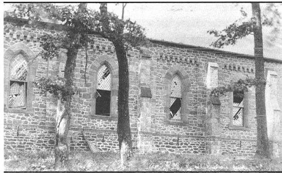
Windows broken in Christ Church after 1890 explosion Taken October 7, 1890
