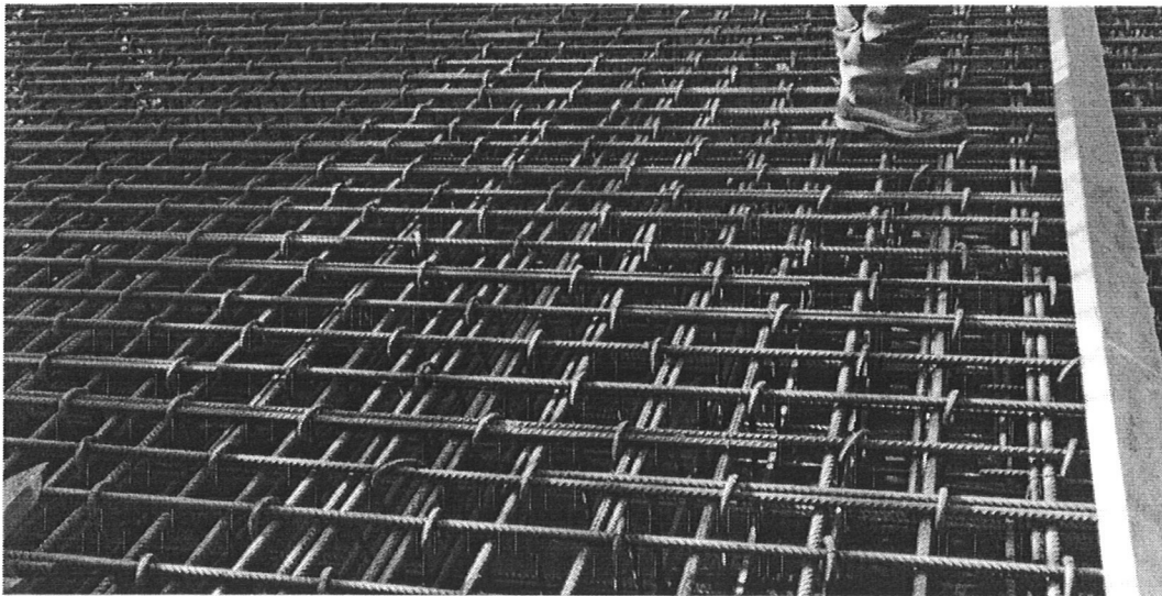
Figure 6: Reinforcement bars in the roof of a cell structure, before cement pouring.
