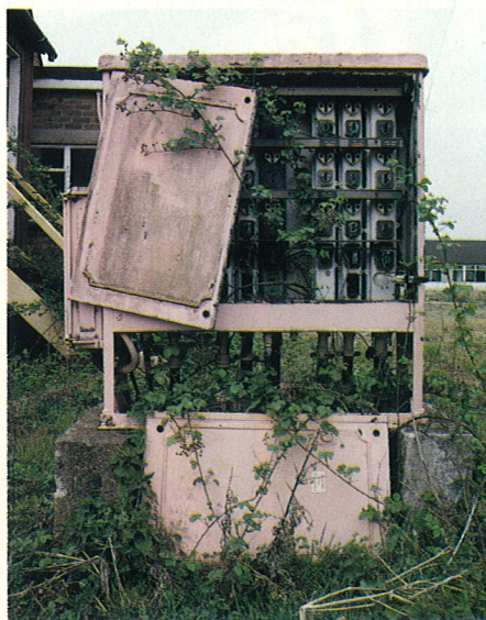
Top: the Grade I-listed Incorporating Mills, 1861. Above: vegetation invades a switchboard
