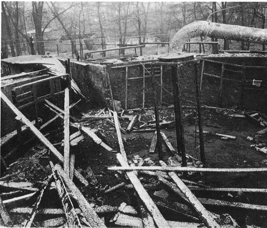
Just 200 feet to the south of No. 18 lay the old dry Stove No. 19. The wooden structure caught fire, this picture giving a good illustration of the method of constructing the inner building inside the protective mound. The view is looking west across the truck line, towards No. 14 Stove and the Engine House.
