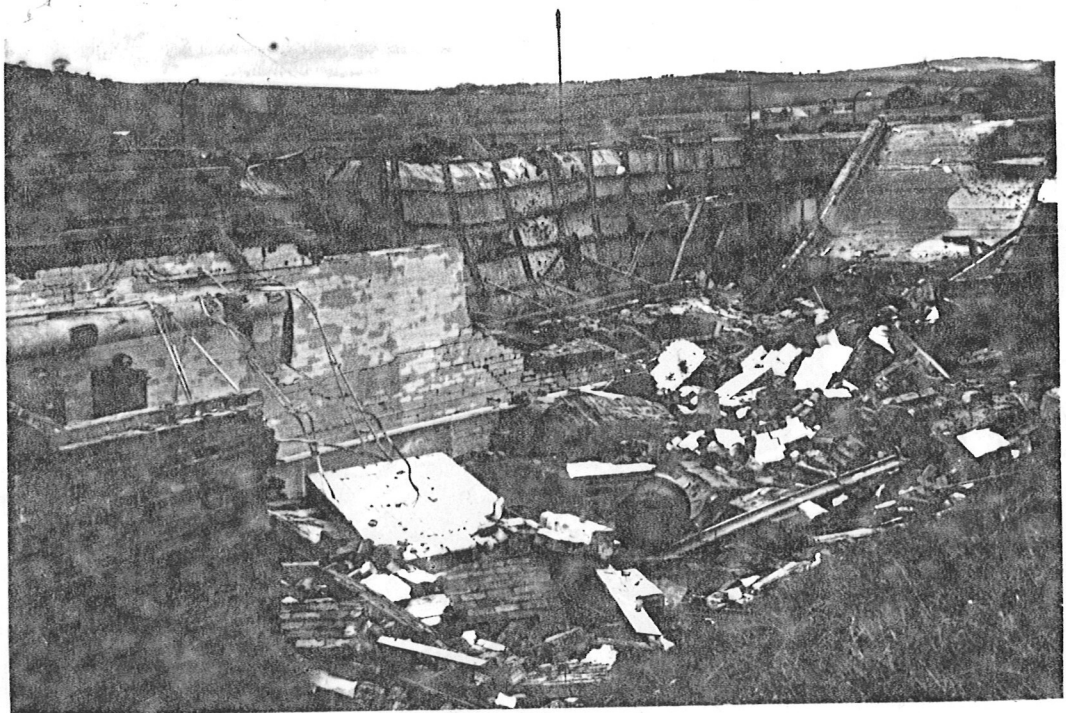
View showing roof collapsed on floor of bay 3. VIEW FROM BACK OF HOUSE LOOKING S.
