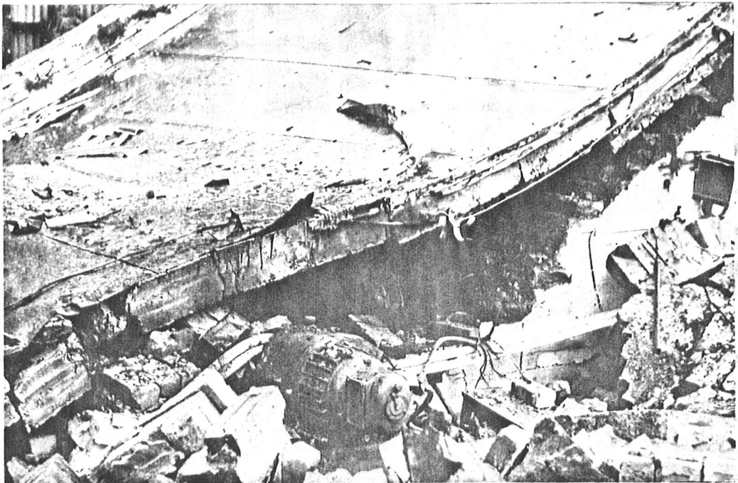
View showing roof collapsed on floor of bay 3.
