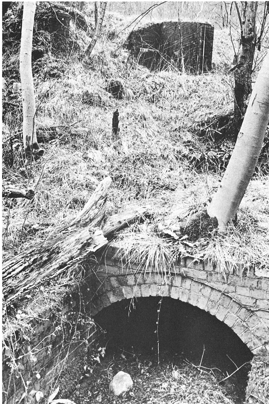
In the background is the building which housed the Pelton wheel. The foreground shows the culvert for run-off water from the wheel
