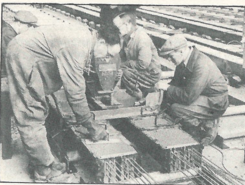
Above: Concrete having been poured, the surfaces of the reinforced sleepers are being trowelled (left); this done, the castings are then vibrated to remove air bubbles and consolidate the mix. These three pictures are examples of how skills could be applied in a diversity of work to retain employment until munitions requirements and weapon development picked up again
